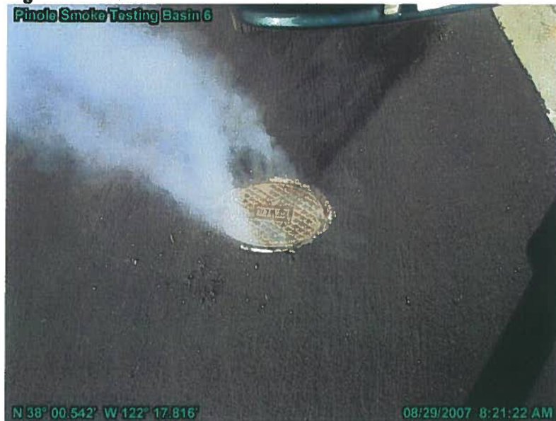
Figure 6-5 Manhole with inflow defect
