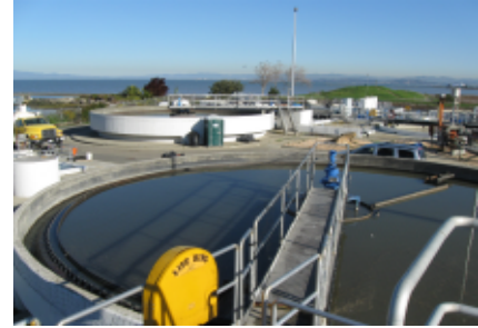
Primary Clarifier No. 1
