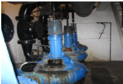
Influent Pumping Station
