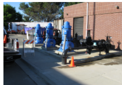
Effluent Pump Station
