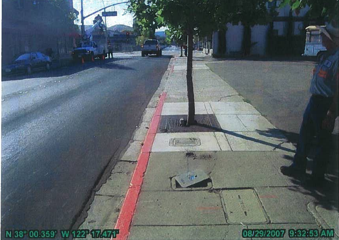
Pinole Smoke Testing Basin 6 Defect 27 - 660 Tennent - Cleanout @ sidewalk
