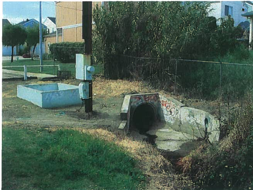
Figure 6-10 Hazel Street Pump Station
