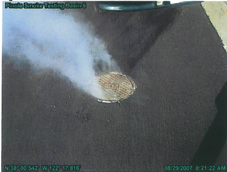
Figure 6-5 Manhole with inflow defect
